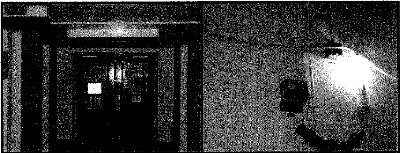
Figure 12: Door separating Building 707 and Building 776/777 with detector mounted just behind. Detector for Building 707 (mounted in Building 776/777) that was inadvertently removed.
