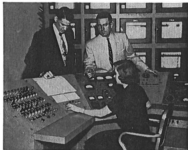
Figure 19. NCSC reactor console
